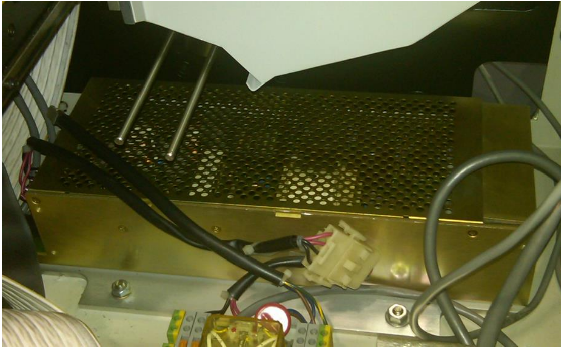
Fig. 61 – 24V Power Supply (Older style)
